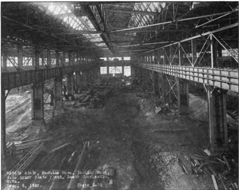
Main aisle of machine shop, Armor Plant, Charleston, W. Va.
