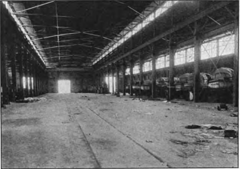
Partial interior view, boat and general storage building, Navy Yard, Philadelphia, Pa.
