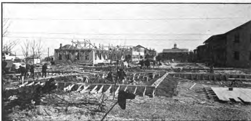
Barracks and mess-hall, Naval Air Station, Hampton Roads, Va. ; view of court.
